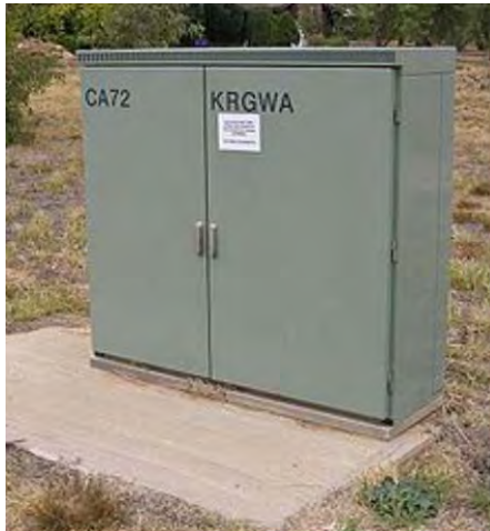
Telstra will upgrade its curb-side equipment to provide better broadband services.
